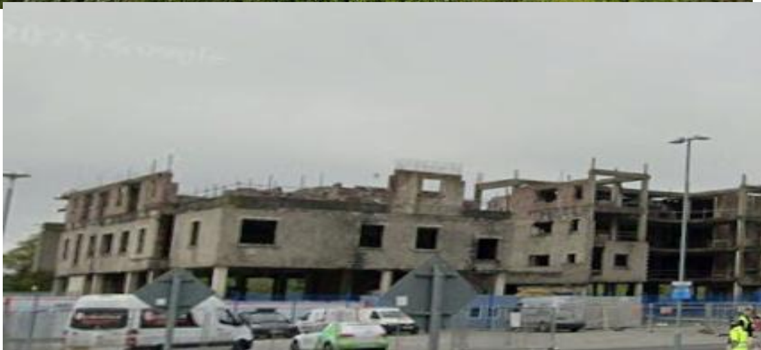
Photograph of unfinished structure (Green Star) which will provide a mix of community, retail, and office space for the area.
